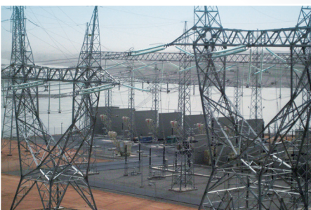
Sudan Merowe Dam 7 autotransformers 50 MVA - 500 kV 2009
